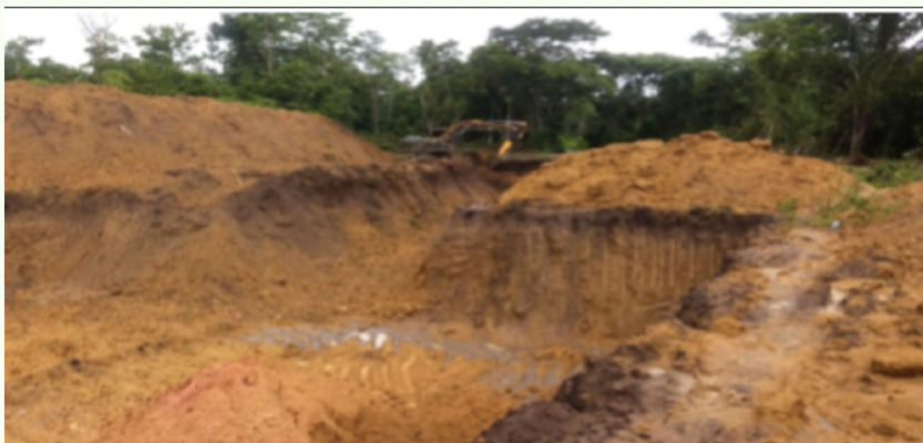
Image 2 - Holes dug by hydraulic backhoes that dig the banks of the rivers in search of gold and destroy the riparian forests.
